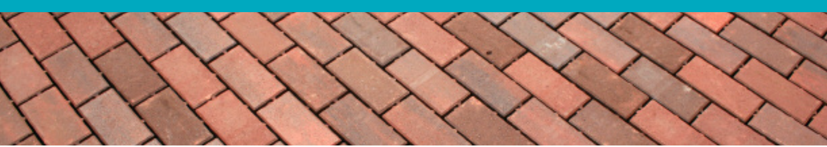
Concrete pavers along Hillside road allow runoff and snow melt to infiltrate.
