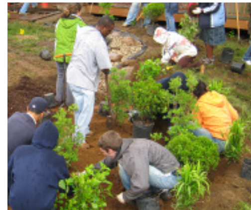
NEMO, with the Horsley Witten Group, conducts a rain garden construction training in Bridgeport, CT.
