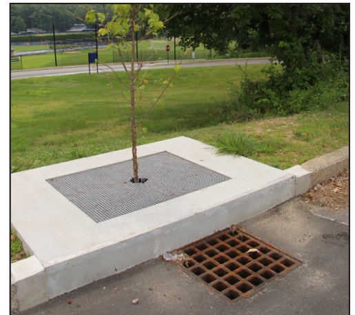
The new MS4 permit emphasizes low impact development practices such as this tree box installation on the UConn campus.
